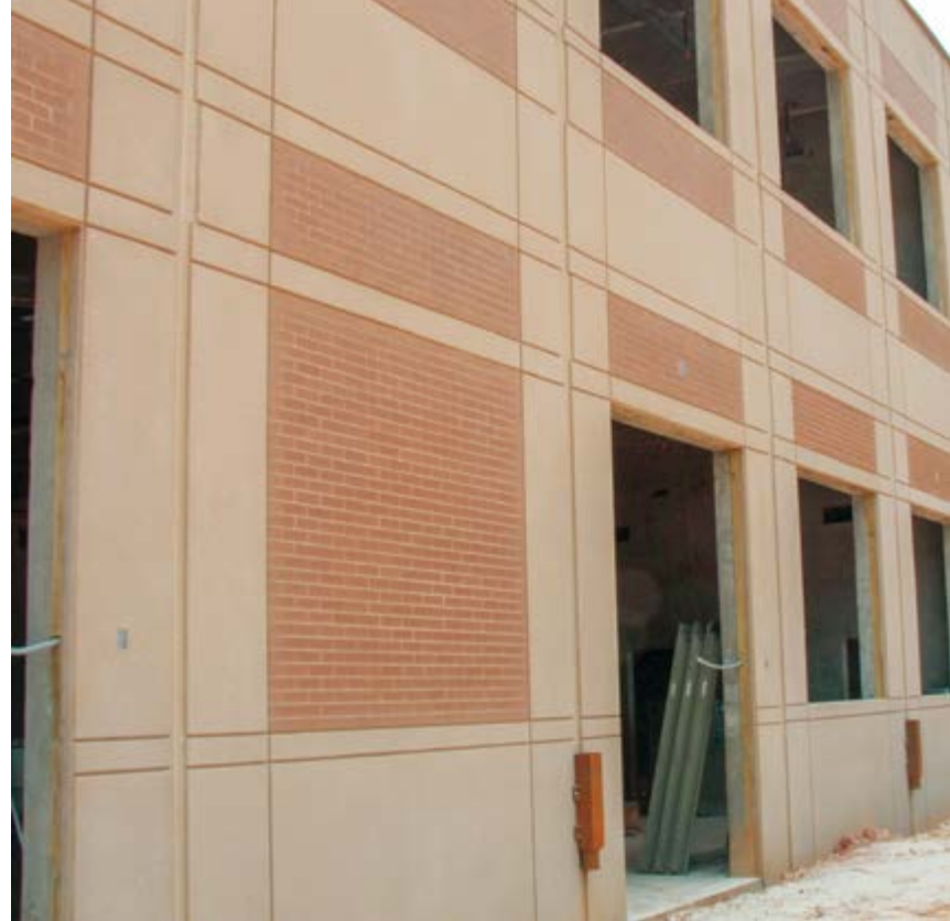
The Eastern Guilford High School design allowed more thin brick to be inset into panels than at Northern Gilford, providing more accents and a warmer appearance.
