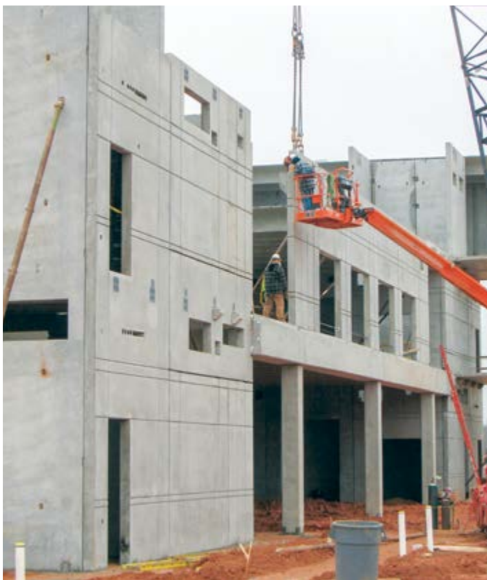
The total-precast concrete structural framing system allowed Eastern Guilford High School to be erected quickly, helping to meet an aggressive schedule after the original building was destroyed. Photo: Tindall Corp.
